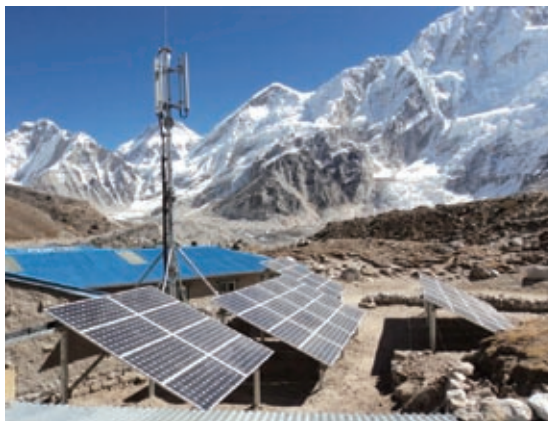
■ Base station with the highest altitude in the world built by the Group
